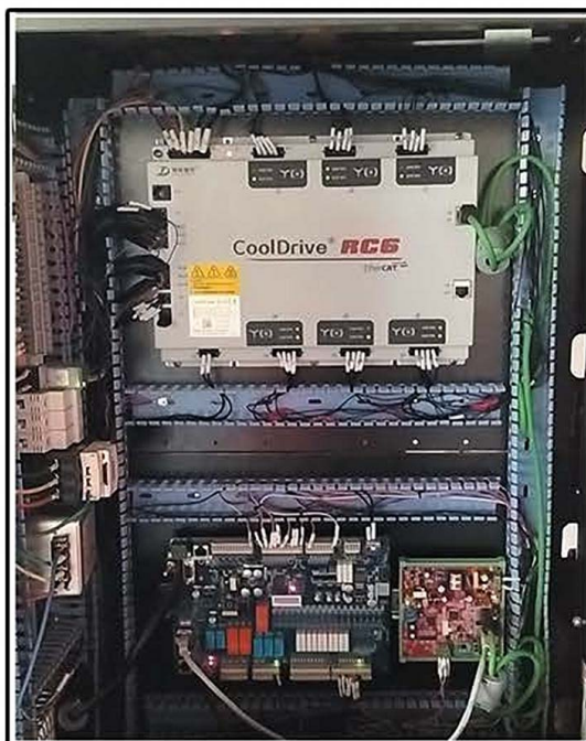
Yooheart New Control Cabinet Inside Design
